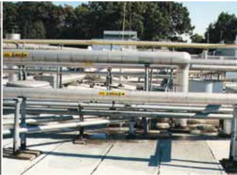
Excessive Roof Loading
